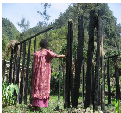
A resident of Wuangima with the charred remains of her house, Porgera, Papua New Guinea, 2009.
